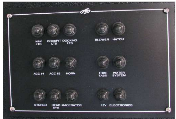
Main Helm Switch Circuit Breaker Panel
