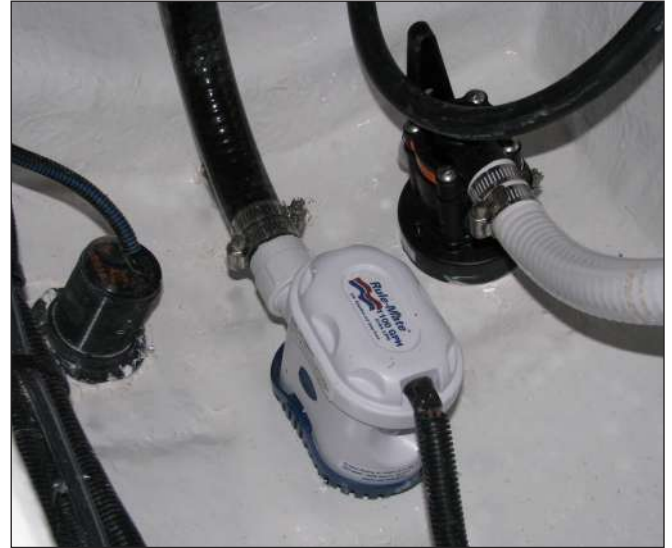
Typical Bilge Pump with Automatic Float Switch
