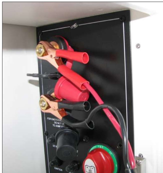
Jumper Harness Connected To Terminals
