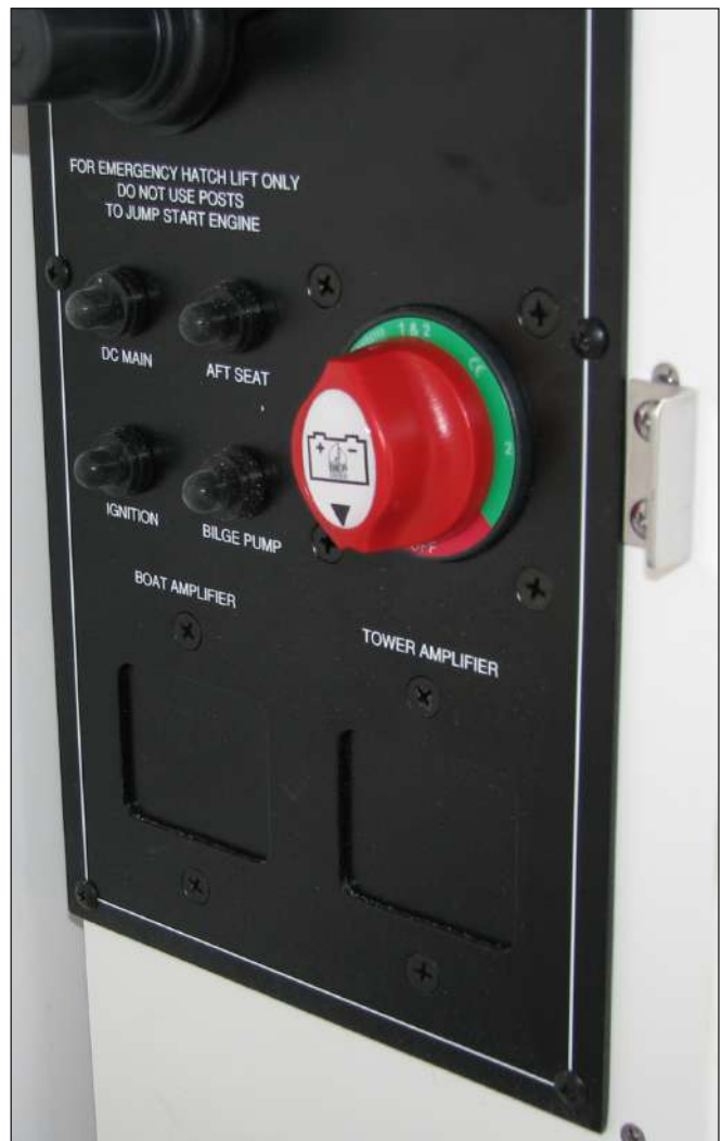
Battery Switch Panel Circuit Breakers
