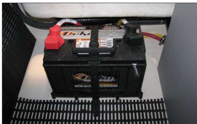
268SS Battery Installation
