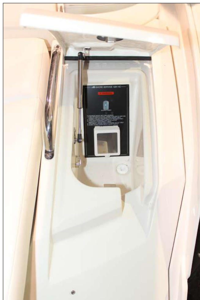
328SS Shore Power Inlet Panel
