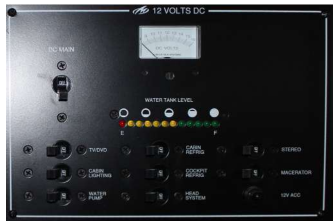
Cabin DC Electrical Panel
