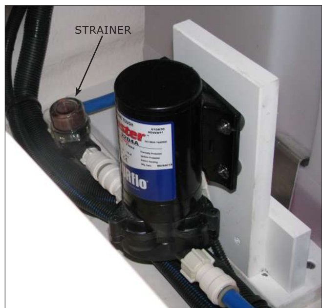
Typical Water Pump & Strainer
