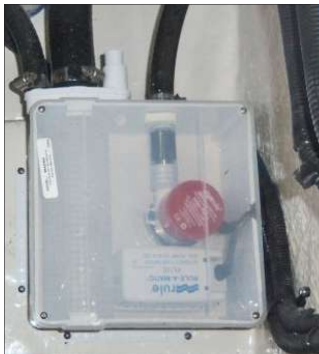
Sump Pump System
