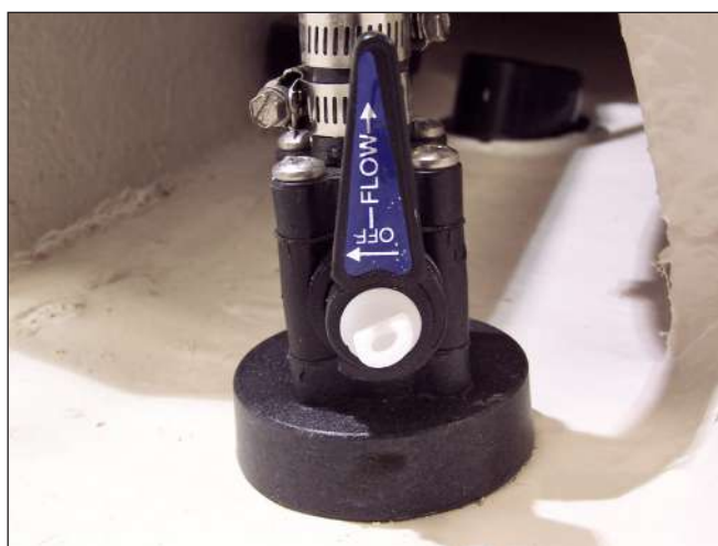
Air Conditioner Seacock (Thru-Hull Valve)
