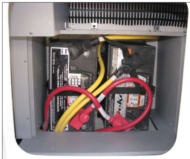
288SS Battery Installation Below Port Stern Seat
