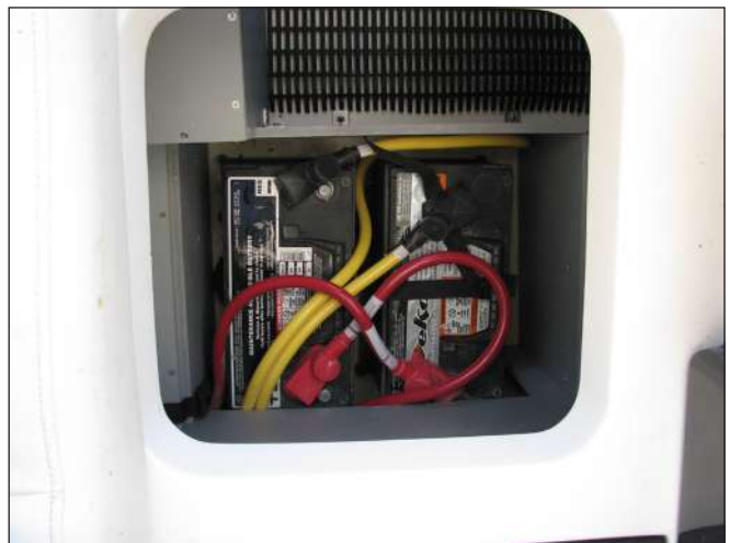
288SS Batteries In Aft Bench Seat Compartment
