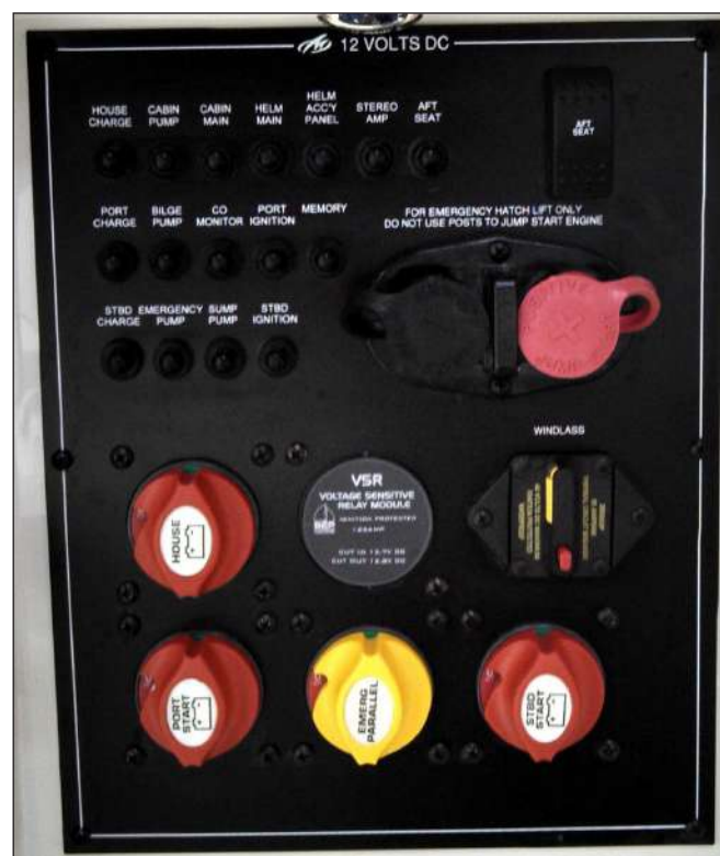
328SS Battery Switch Panel
