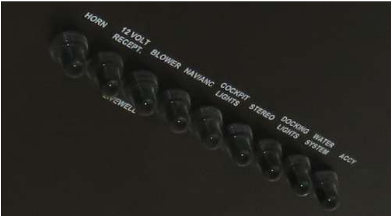
Helm Accessory Circuit Breaker Panel
