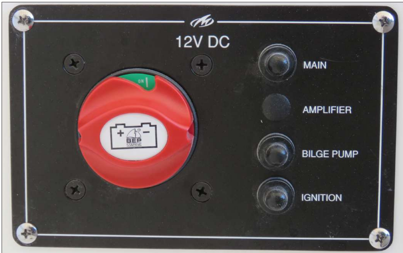
Battery Switch & Circuit Breakers
