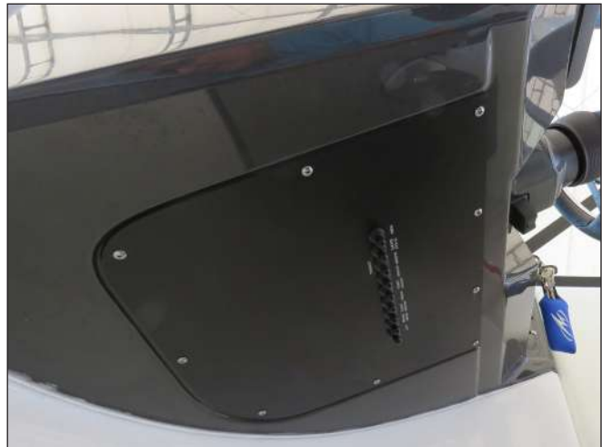
Removable Circuit Breaker Panel
