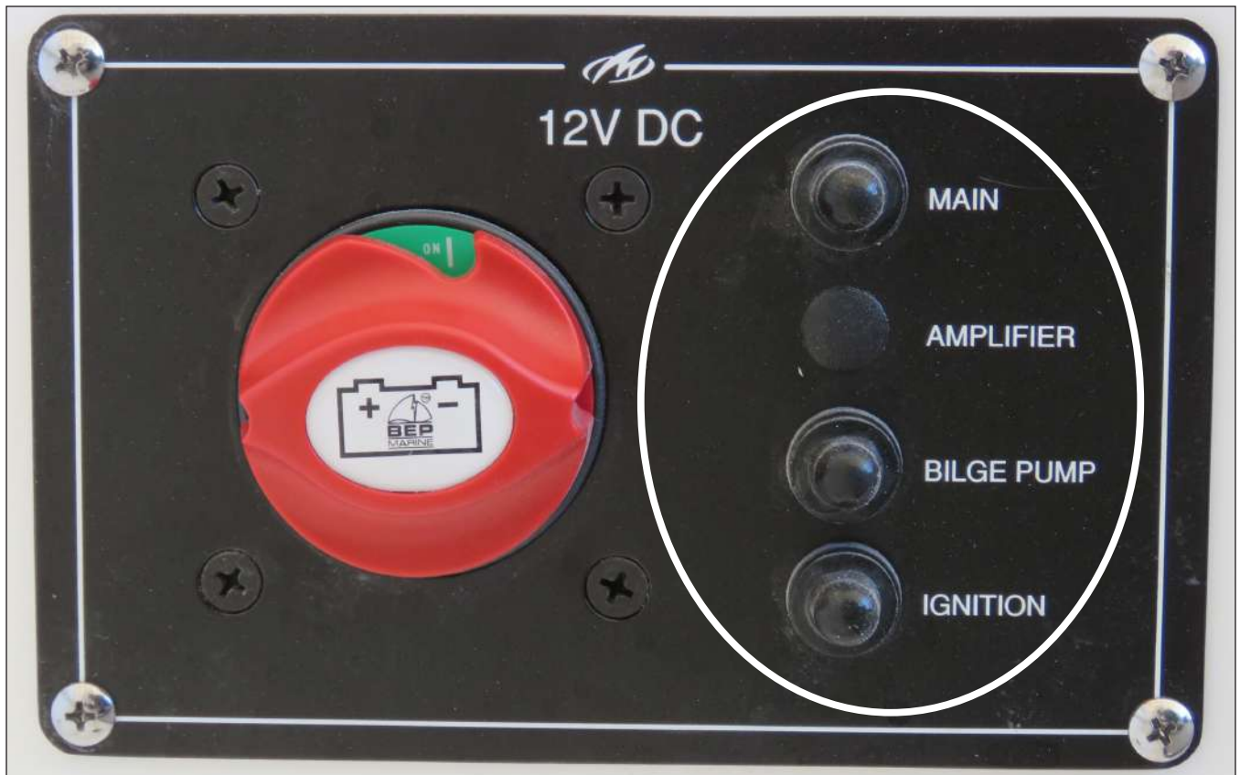
Battery Switch Panel Circuit Breakers
